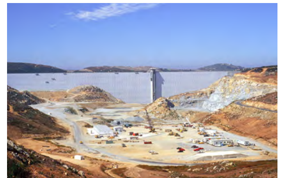
Most construction activity took place on the floor of the future reservoir. Working within this small space preserved the surrounding natural resources.
